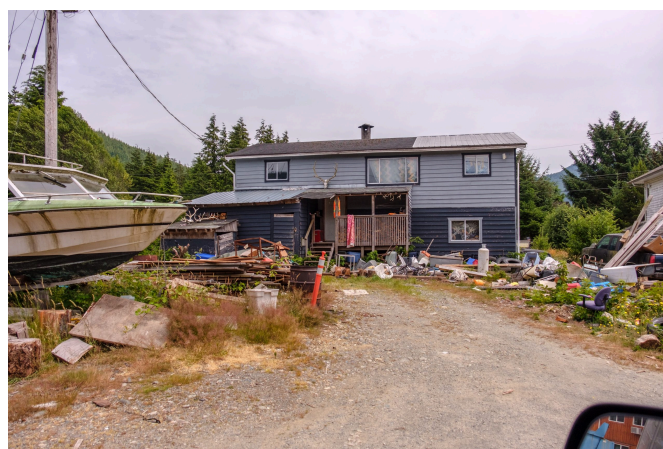
House in need of serious repair, Malachan Indian Reserve, Vancouver Island (2017) Credits to: Mikofox Photography (CC BY-NC-SA 2.0) [135]
