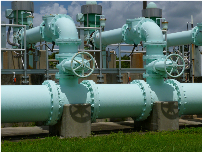
Gas Pipe Control Station, Blue Heron Wetlands. Credits to: Rusty Clarke (CC BY 2.0) [172]
