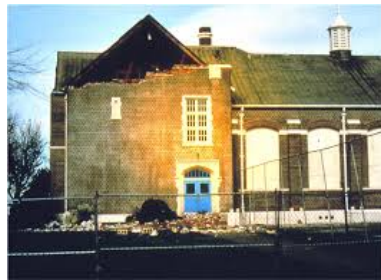
Figure 14-3. Damage to Molalla High School, an unreinforced-masonry (URM) building, from the Scotts Mills Earthquake of 1993. Bricks from the URM gable over the doorway fell on the steps and sidewalk. Fortunately, the earthquake occurred early in the morning, and no students were in the building. Photo courtesy of Yumei Wang, Oregon Department of Geology and Mineral Industries
