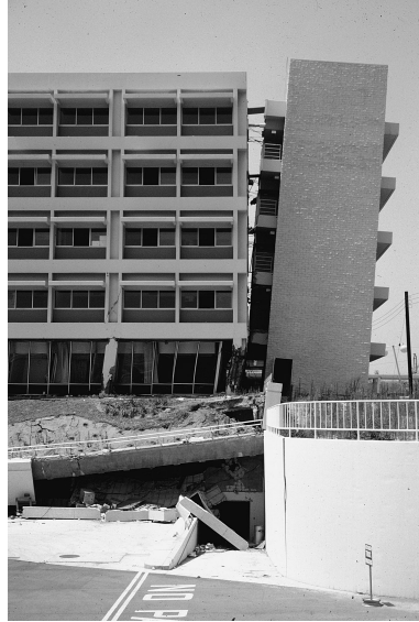
Figure 12-10. Damage to the Los Angeles County Olive View Medical Center as a result of the 1971 Sylmar, California, Earthquake. The first floor, with a lot of open space, behaved like a soft story, causing the upper floors to move relatively to the right, forcing out the stairwell. Photo by Robert Yeats
