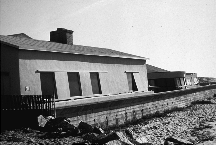
Figure 8-6. Tilted buildings at San Jose State University Marine Laboratory at Moss Landing, California, due to liquefaction of beach deposits during the October 1989 Loma Prieta Earthquake. Photo by G. W. Wilson, USGS
