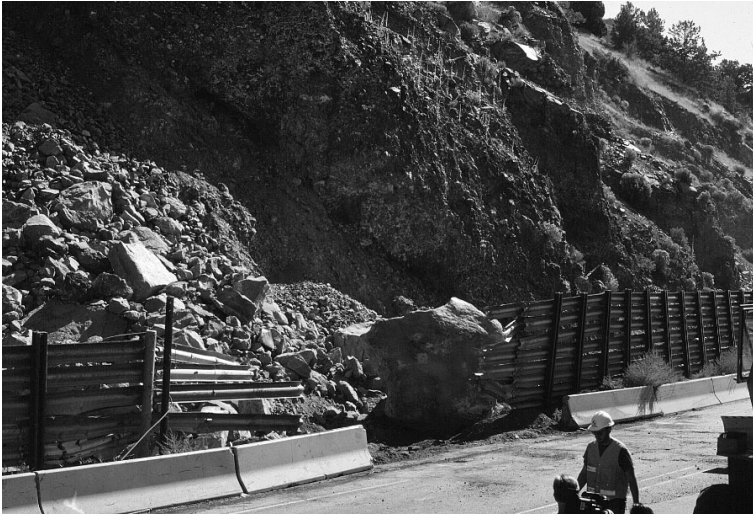
Figure 6-24. Boulder at Modoc Point, alongside U.S. Highway 97, that breached a roadside barrier and took the life of Ken Campbell during the September 20, 1993, Klamath Falls Earthquake. Boulder has been pushed back behind barrier.
