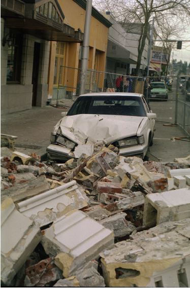
Figure 5-7. Parapet failure on the south side of the Washington Federal Savings building in downtown Olympia as a result of the 2001 Nisqually Earthquake. Downtown Olympia is built on several hundred feet of latest Pleistocene sediments, which amplified seismic waves. Photo by Joe Dragovich, Washington Division of Geology and Earth Resources.
