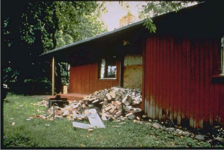
Figure 11-13. Brick chimney on this house in Petrolia, California, collapsed during the 1992 Cape Mendocino Earthquake. Photo courtesy of National Oceanic and Atmospheric Administration
