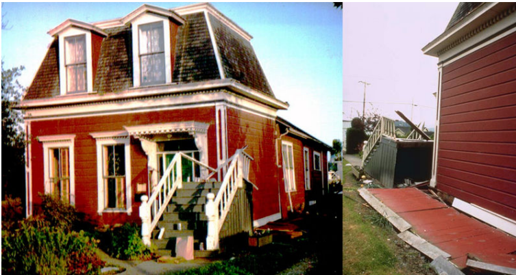
Figure 11-4. This Victorian wood-frame house in Ferndale, California, was built on a post-and-pier foundation, but was not bolted to its foundation, so that it slid off during the 1992 Cape Mendocino Earthquake. The floor level of the house was at the same height as the front steps. The house moved to the right and down with respect to the steps. The wooden skirting, formerly part of the outside wall, is now flat on the ground. Left-hand photo is view of house from front, and right-hand photo is view from one side. Photos courtesy of National Oceanic and Atmospheric Administration
