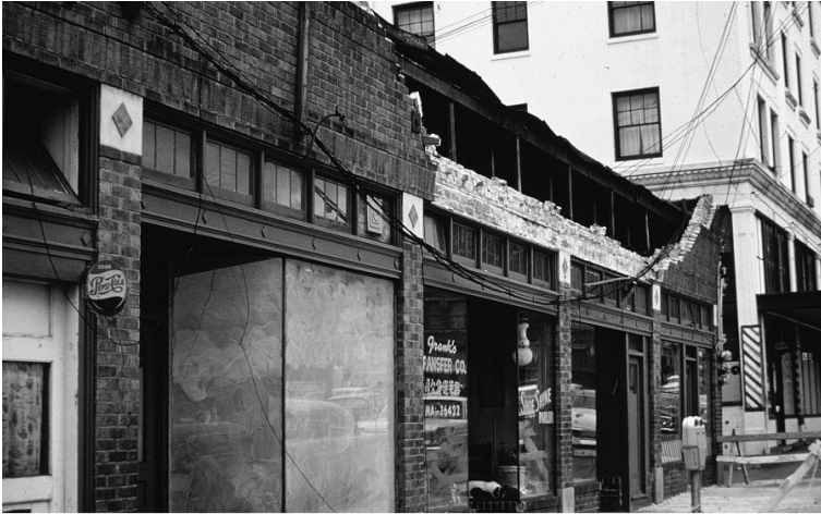
Figure 5-6. Falling bricks from this building on King Street, Seattle, during 1965 earthquake caused one death. From Karl V. Steinbrugge Collection, Photo 2876
