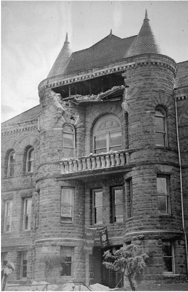
Figure 5-4. Damage to Old State Building, Olympia, Washington, in 1949 earthquake. From Thorsen (1986); illustration from collection of Washington Division of Geology and Earth Resources
