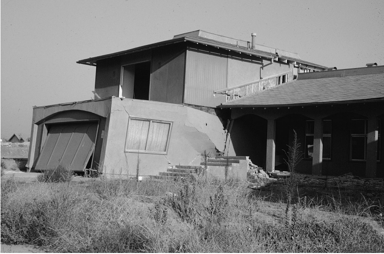
Figure 11-16. Split-level house in Crestview Tract, San Fernando Valley, showing failure of the connection between the single story (right) and the two-car garage with bedrooms above. Note the difference in height between the front steps and the single story, indicating cripple-wall failure of the single story. Photo by Robert Yeats
