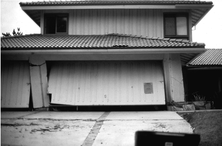
Figure 11-6. Soft-story failure to three-car garage during 1971 Sylmar, California, Earthquake. The large door opening resulted in inadequate shear resistance to horizontal ground motion. Photo by J. Dewey, USGS
