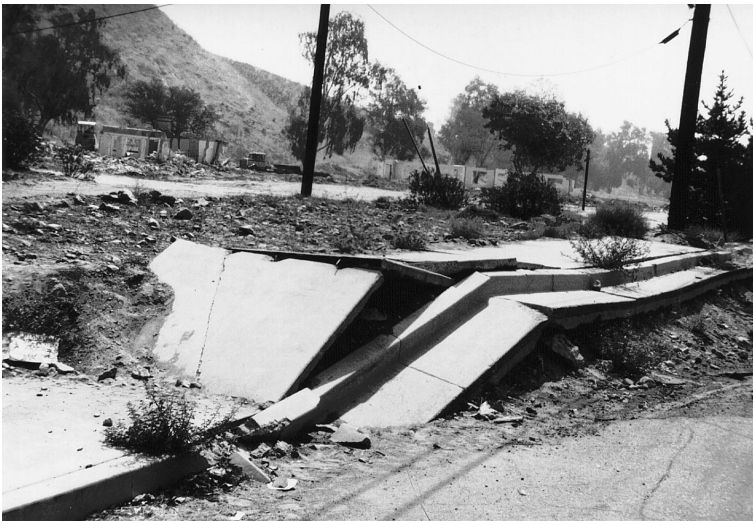
Figure 3-8a. Reverse fault in the San Fernando Valley, California, formed during the Sylmar Earthquake of February 9, 1971. Fault extends from left to right. Buckling of sidewalk indicates compression; fault dips away from viewer. Hanging wall (in background) was at same level as footwall (in foreground) before the earthquake. Ruined building in left background was part of a convalescent home in which several people died.
