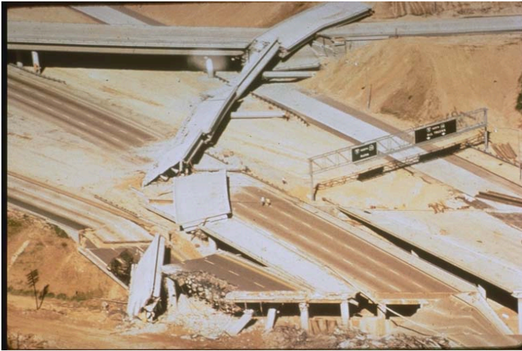
Figure 12-14. Damage to the Golden State Freeway (Interstate 5) and Foothills Freeway (Interstate 210) as a result of the 1971 Sylmar, California, Earthquake. Photo by E. V. Leyendecker, USGS
