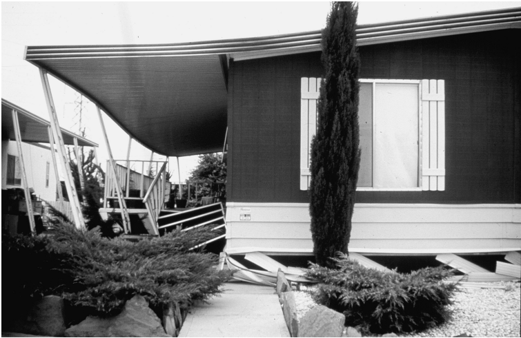
Figure 11-17. This manufactured home slipped off its supporting piers during an earthquake. This type of failure can be avoided by bolting the house to its foundation, as is required for other houses in most states. From Karl Steinbrugge Collection, University of California at Berkeley
