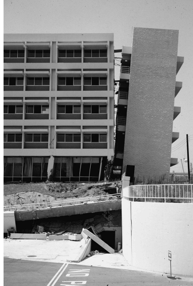
Figure 12-10. Damage to the Los Angeles County Olive View Medical Center as a result of the 1971 Sylmar, California, Earthquake. The first floor, with a lot of open space, behaved like a soft story, causing the upper floors to move relatively to the right, forcing out the stairwell. Photo by Robert Yeats
