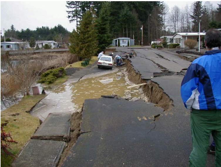
Figure 8-8. Lateral spread at Sunset Lake, Tumwater Memorial Mobile Home Park near Tumwater, Washington. Photo by Steven Kramer, University of Washington.
