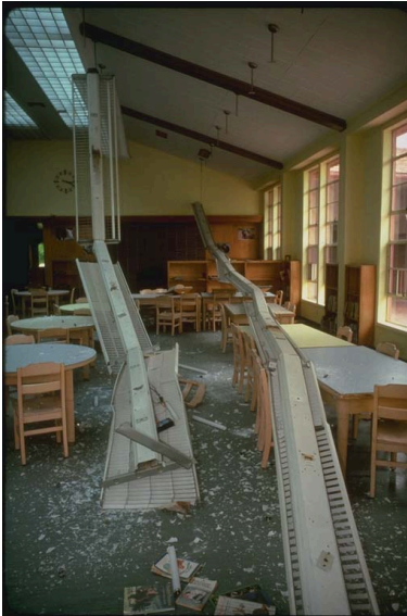
Figure 12-7. Failure of hanging light fixtures at library of Dawson Elementary School in California, fortunately unoccupied at time of earthquake. Note fallen ceiling tiles and plaster. Photo credit: Earthquake Engineering Research Institute
