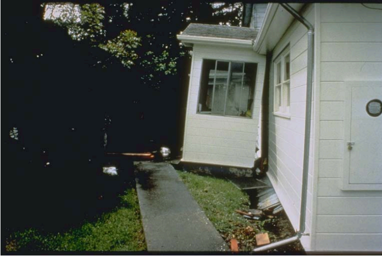
Figure 11-5. This house south of Petrolia, California, shifted off its foundation during the 1992 Petrolia Earthquake because it was not anchored to the foundation, and its cripple wall was not reinforced. The house shifted to the right, as seen by the collapsed wooden skirting. The separation of the house and the small porch is an example of connection failure. Photo courtesy of National Oceanic and Atmospheric Administration
