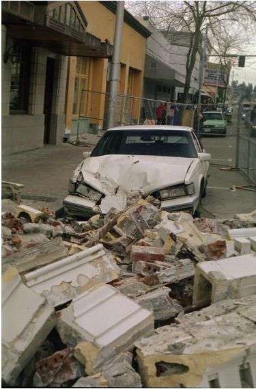
Figure 5-7. Parapet failure on the south side of the Washington Federal Savings building in downtown Olympia as a result of the 2001 Nisqually Earthquake. Downtown Olympia is built on several hundred feet of latest Pleistocene sediments, which amplified seismic waves. Photo by Joe Dragovich, Washington Division of Geology and Earth Resources.
