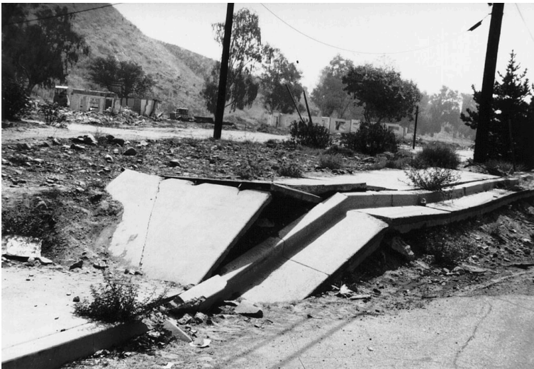
Figure 3-8a. Reverse fault in the San Fernando Valley, California, formed during the Sylmar Earthquake of February 9, 1971. Fault extends from left to right. Buckling of sidewalk indicates compression; fault dips away from viewer. Hanging wall (in background) was at same level as footwall (in foreground) before the earthquake. Ruined building in left background was part of a convalescent home in which several people died.
