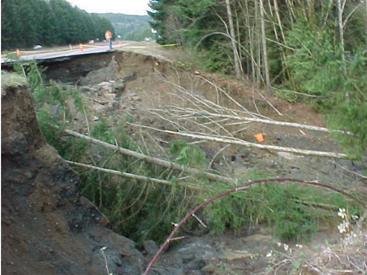
Fig. 8-13. Landslide across Highway 101, about 100 feet across. Photo courtesy of Jon Bray, University of California Berkeley.
