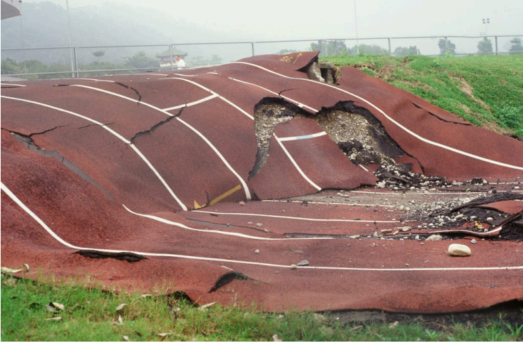
Figure 3-8b. Reverse fault across a running track at Kuangfu High School in central Taiwan, formed by Chelungpu reverse fault during Chi-Chi earthquake. Photo by Robert Yeats for both 3-8 a and b.
