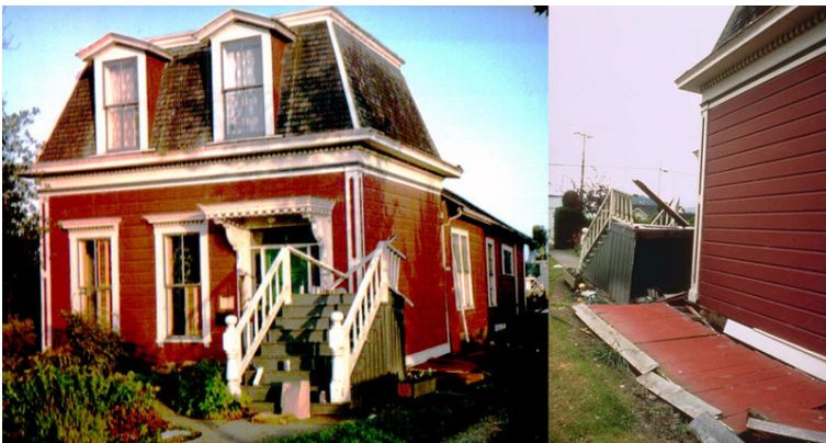
Figure 11-4. This Victorian wood-frame house in Ferndale, California, was built on a post-and-pier foundation, but was not bolted to its foundation, so that it slid off during the 1992 Cape Mendocino Earthquake. The floor level of the house was at the same height as the front steps. The house moved to the right and down with respect to the steps. The wooden skirting, formerly part of the outside wall, is now flat on the ground. Left-hand photo is view of house from front, and right-hand photo is view from one side. Photos courtesy of National Oceanic and Atmospheric Administration
