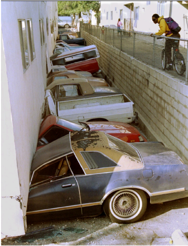
Figure 12-12. Soft-story problem in apartment building where bottom floor is the garage. During 1994 Northridge earthquake, the garage acted as a soft story, and the apartments above collapsed down on the cars.
