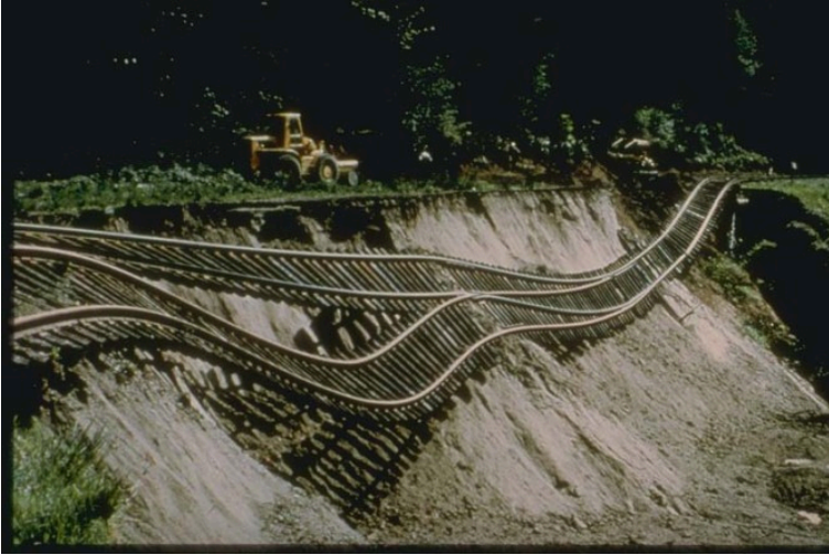
Figure 8-10. Hillside slid away from beneath this four-hundred-foot section of a Union Pacific Railway branch line at Tumwater, near Olympia, Washington, during the Puget Sound Earthquake of 1965. A large landslide during the heavy-rainfall winter of 1996-97 also damaged the rail line. Photo by G.W. Thorsen, Washington Division of Geology and Earth Resources.
