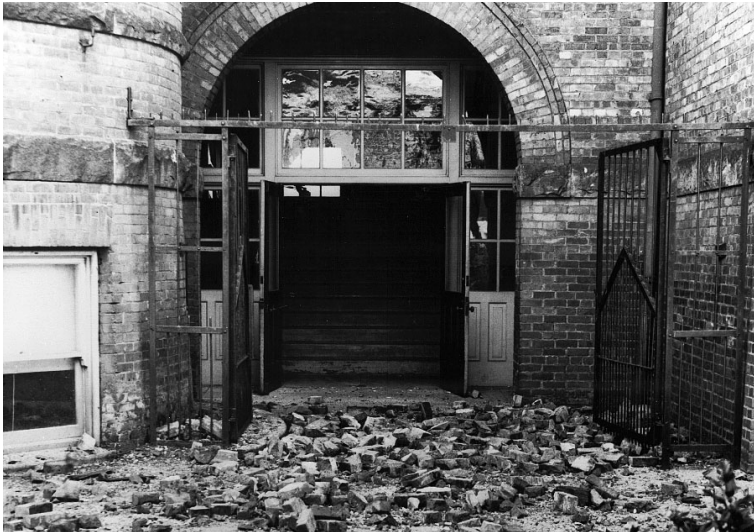
Figure 12-2. Close-up of an entrance to Lafayette School in West Seattle, covered with bricks that fell from this unreinforced masonry building during the 1949 Puget Sound Earthquake. Fortunately, the school was not occupied at the time, and no children were killed or injured. Damage to this and other schools in the 1949 and 1965 earthquakes led to a major retrofit of school buildings that minimized school damage in the 2001 earthquake. Photo courtesy of Washington Division of Geology and Earth Resources.
