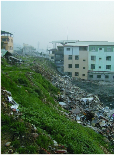
Figure 12-15. The Chi-Chi, Taiwan, earthquake was accompanied by surface rupture on the Chelungpu reverse fault. The photo is taken along the fault with the upthrown hanging wall on the left. The fault trace is between the two buildings in Fengyuan City, on which destruction was total. Photo by Charles Rubin, then of Central Washington University in Ellensburg.
