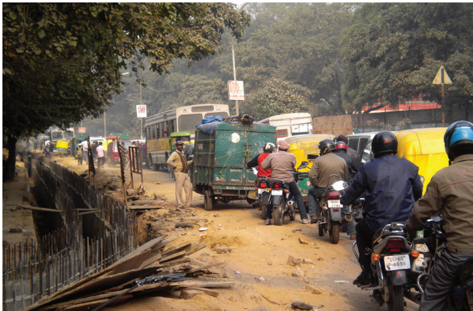
Figure 9.6: Women identified the lack of pavement as severely restricting their mobility and adding to their fear of violence in this area of New Delhi.
