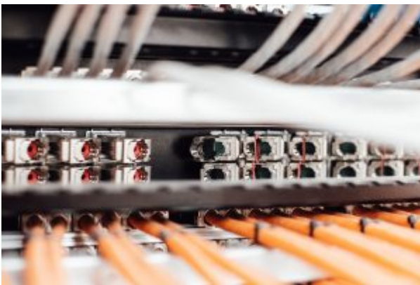
Note. Cable connection, by L. Kienle, 2020.
